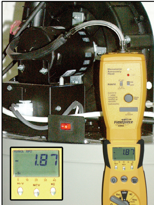
Blocked Vent Switch - Pressure Test Vertex Residential Power Vent Model
